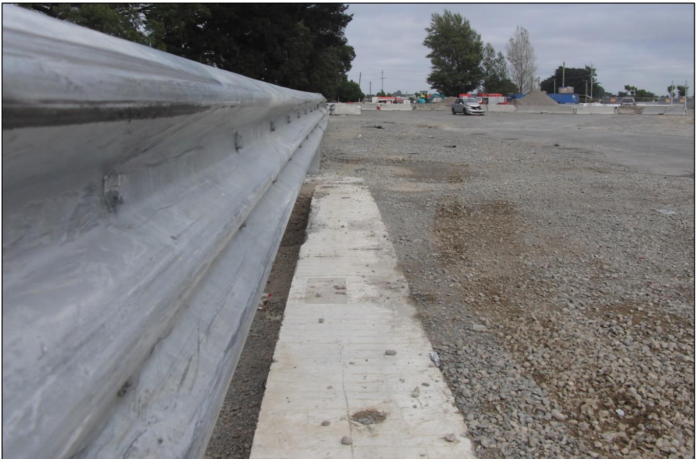
Figure 8: Nil Damage to CrocGuard® Following MASH 4-10 Impact
