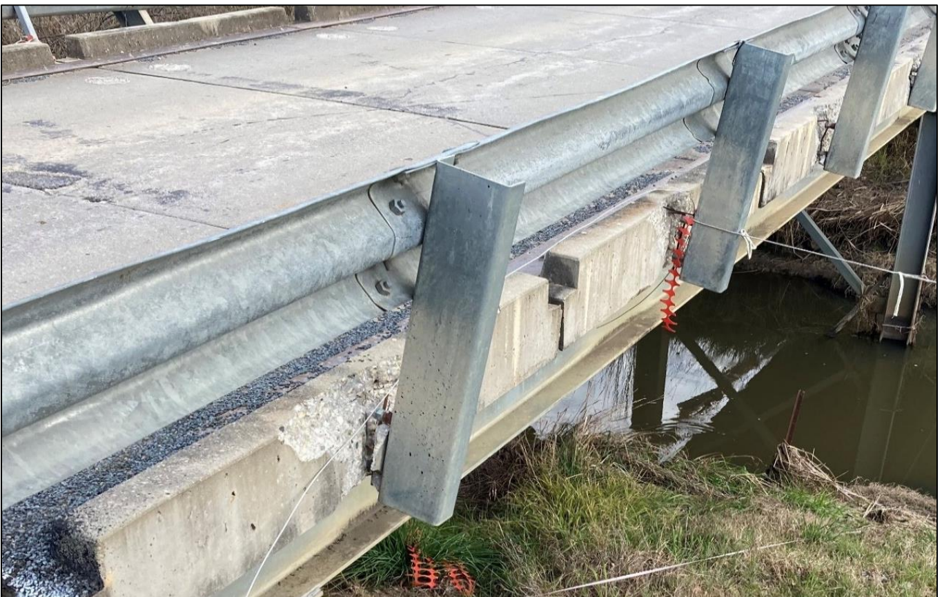
Figure 1: Failure of Rigid Post Systems Causing Significant Damage.
